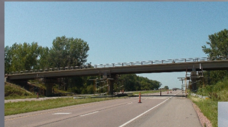
Ben and Doug finished raising 3 bridges in Monona County (south of Sioux City)
