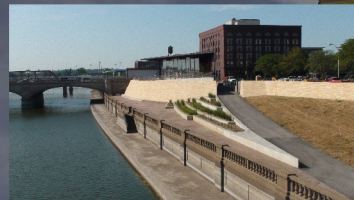
Corps Riverwalk Chuck and Mike V. finished building flood walls in downtown Des Moines. The kiosk building and landscaping is almost done.
