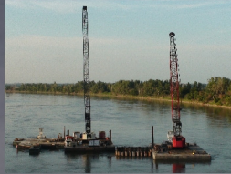
Rulo, NE 1026' x 40' Steel Girder This bridge has really taken off after the slow start in '10-'11. Chad and Nels got it back on track. Now, Chad is finishing Pier 3 and has set some steel girders.
